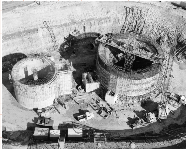
Atlas-F missile silo under construction. Public Domain. The area surrounding the silo would eventually be backfilled to conceal the silo (U.S. Department of Defense archival image. The appearance of U.S. Department of Defense (DoD) visual information does not imply or constitute DoD endorsement.) 21
